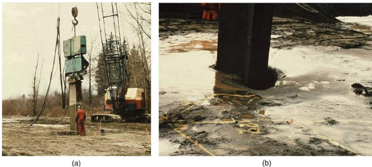
Fig. 5. Resonance compaction and liquefaction of zone around Tri Star probe: (a) compaction equipment; and (b) manifestation of liquefaction during resonance compaction. (Reprinted from Massarsch and Vanneste 1988).
